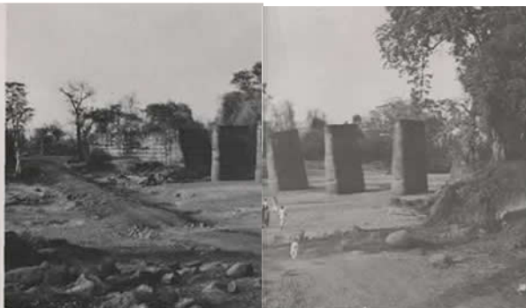
A Tale of Continued Neglect : One of the Many Bridges Left Unfinished
